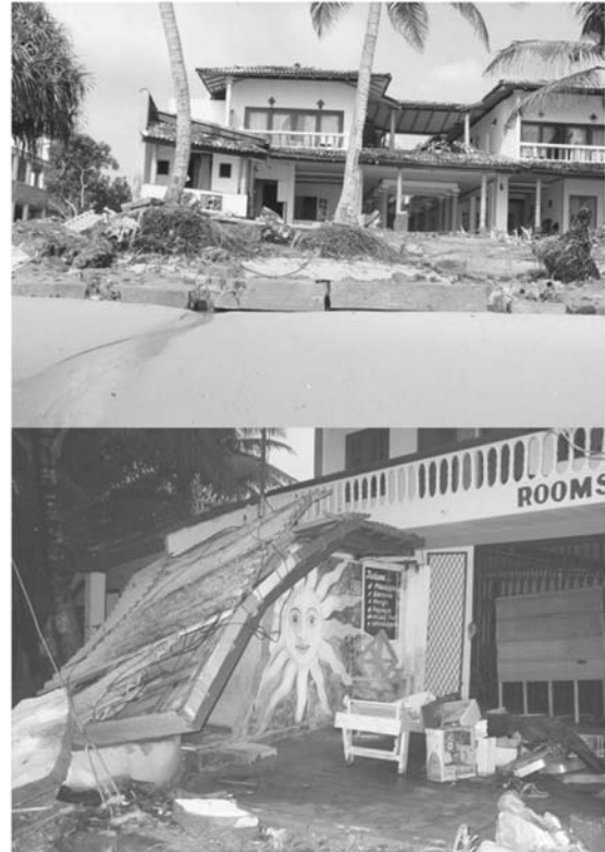
Fig. 3b (Upper) Damaged Tourist hotel and (Lower) Rest-house damaged by tsunami waves
