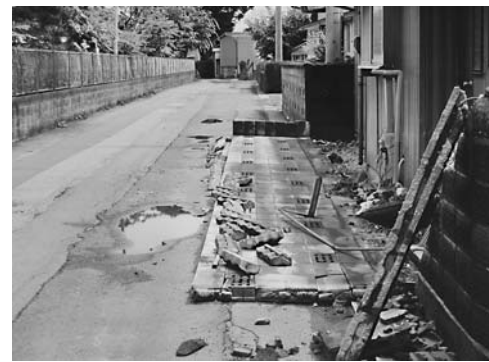
Photo. 5 Fallen concrete block
