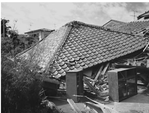
Photo. 3 Collapsed wooden house
