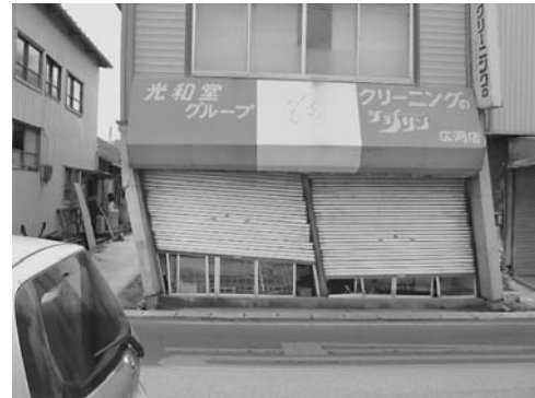
Photo. 4 Damage of pilotis structure
