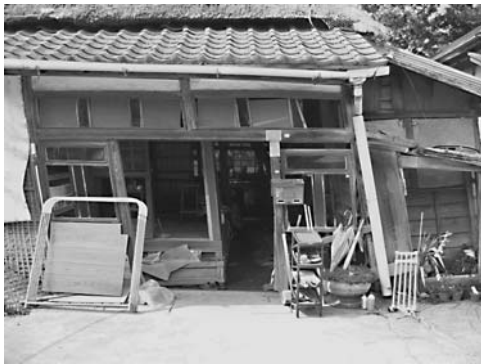
Photo. 1 Severely damaged wooden house
