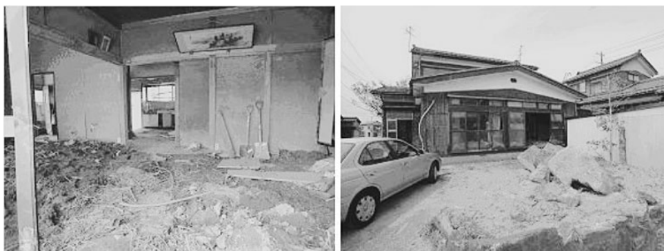
Fig. 14 Damage to the House Closest to the Broken Left Bank of the Ikarashi (Photos by Haruo Hayashi)
